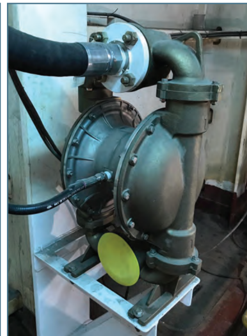
MISTRAL pump 3" for brine circulation, offshore platform (Asia)
